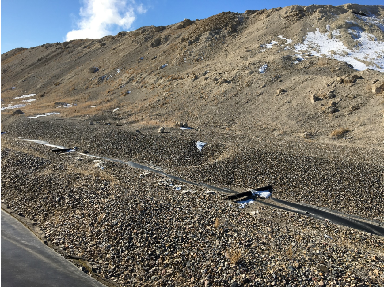
Photo 15. Underdrain collection system, Cell 1 East Side - View Southwest
